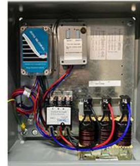
50KA (Motor Protection)
