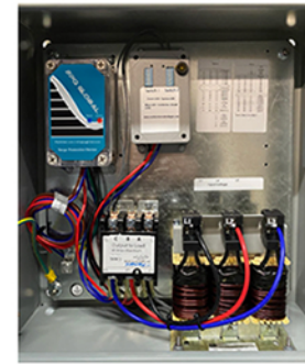
50KA (Motor Protection)
